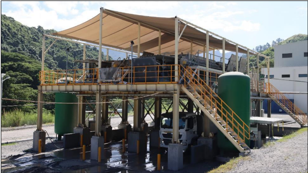
Figure 17.12 Filtration Plant with Two Plate and Frame Filters, Separate Air Compressors for Each Filter and Filter Cake Truck Loadout
