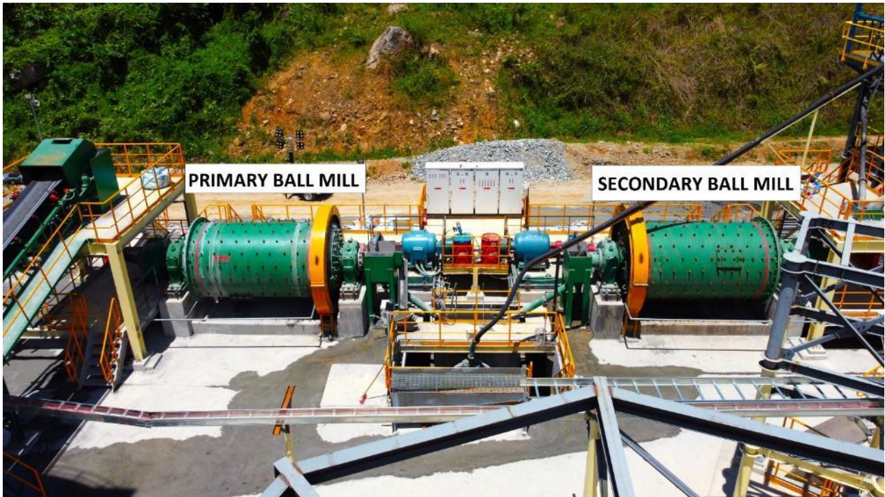
Figure 17.4 Aerial Photograph of the Grinding Circuit
