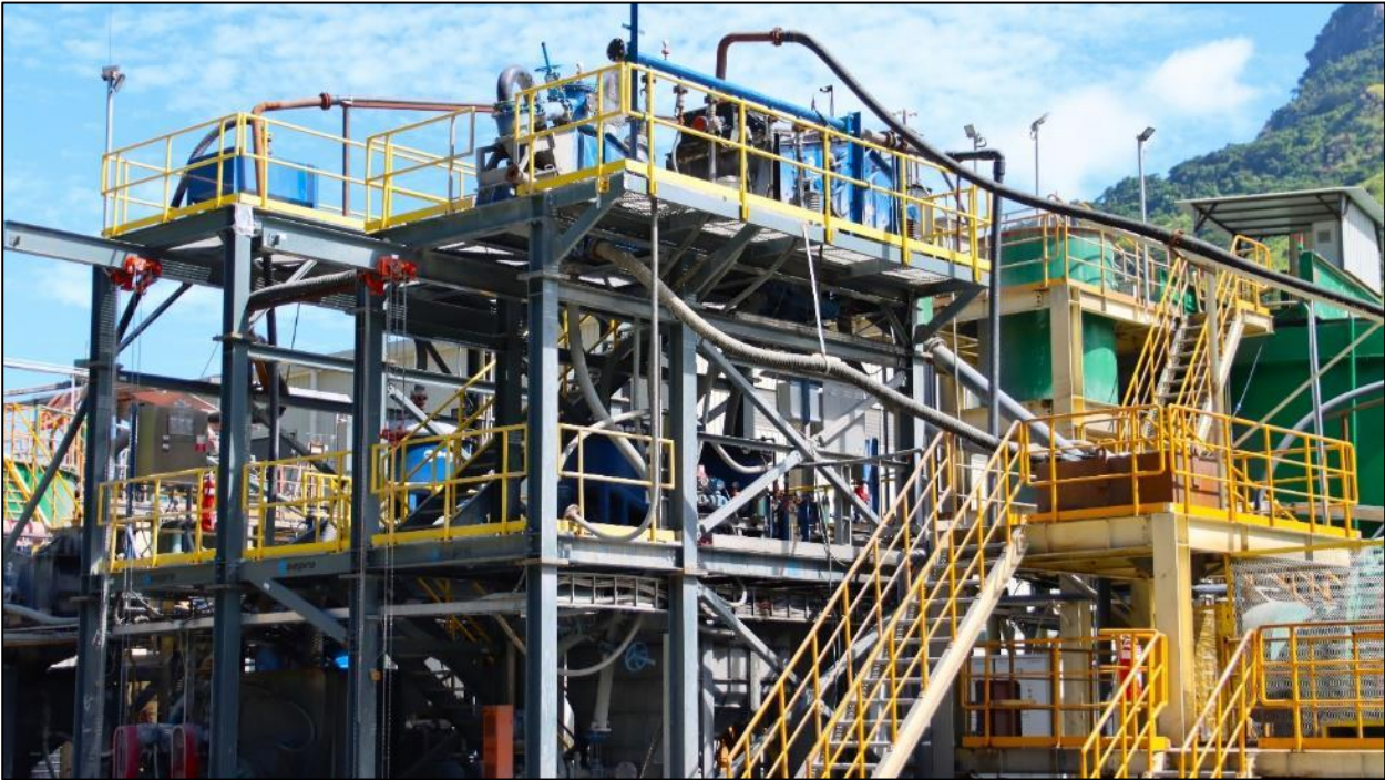
Figure 17.5 Gravity Separation Modules
