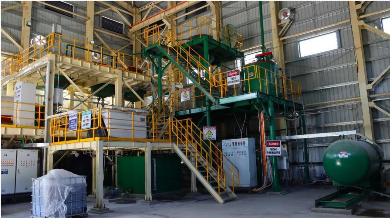
Figure 17.8 The Elution (upper background), Main Pressure Electrowinning Pressure Vessel (far right) and Atmospheric Electrowinning (white tank on the left)
