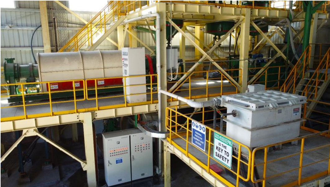
Figure 17.11 Carbon Regeneration Kiln (upper left) and Atmospheric Electrowinning Cell (to the left)
